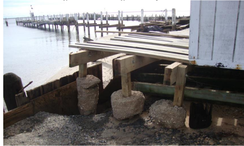
Figure 11: Damages at Bryant Park
